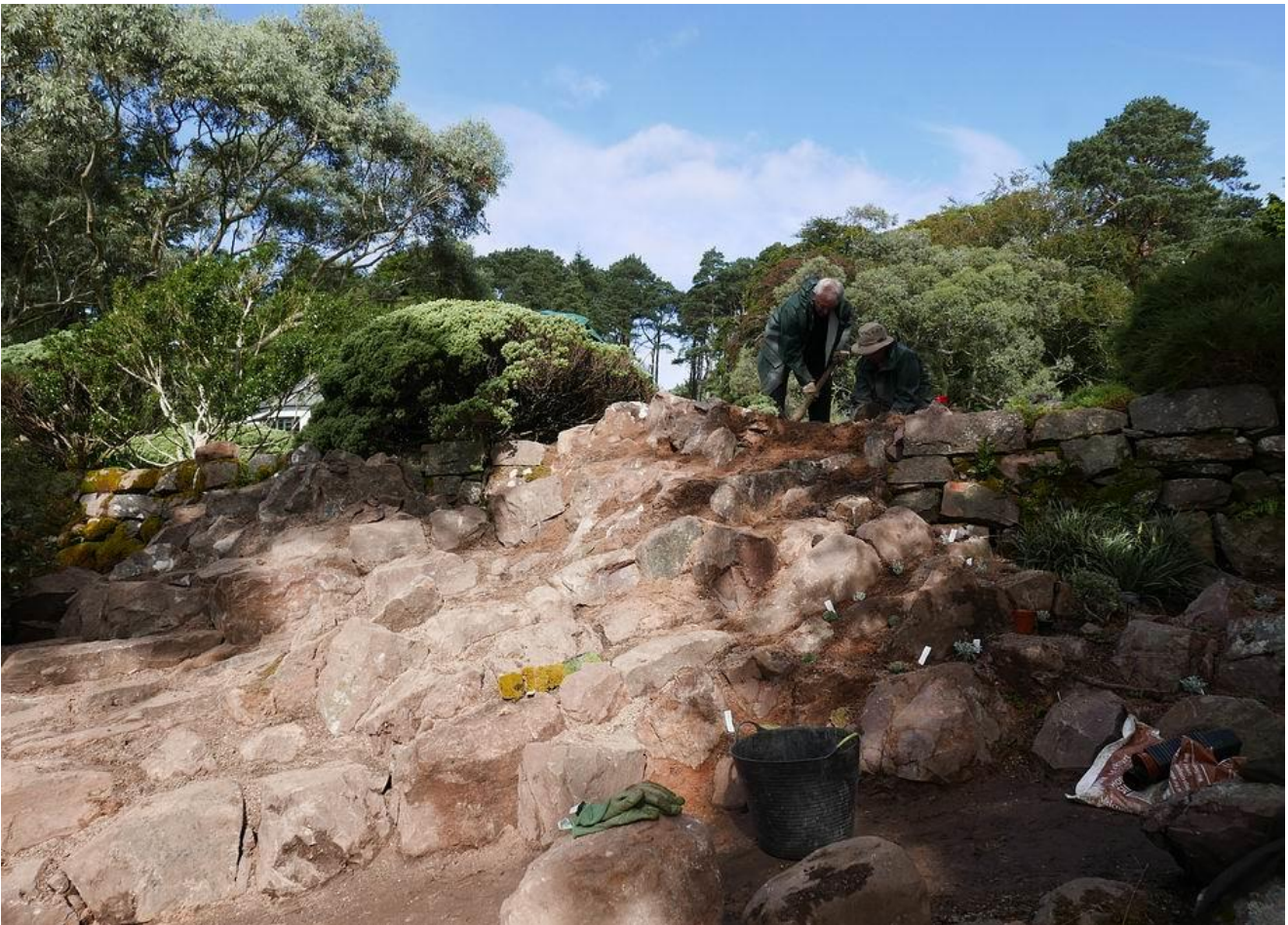
On Friday we had the most magnificent weather with bright blue skies and by the end of the day the construction had moved to the top level.
