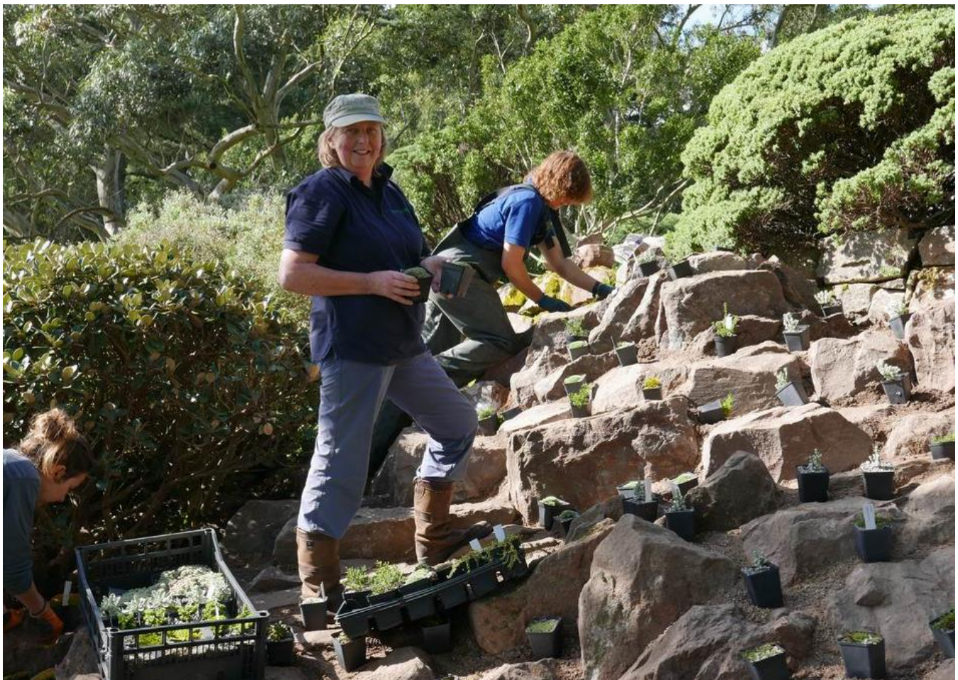
As the construction team completed the lower section we handed it over to Julia Corden who was in charge of both the acquisition and the planting of the plants which, as per the brief from Inverewe, consisted mostly of New Zealand alpine plants.
